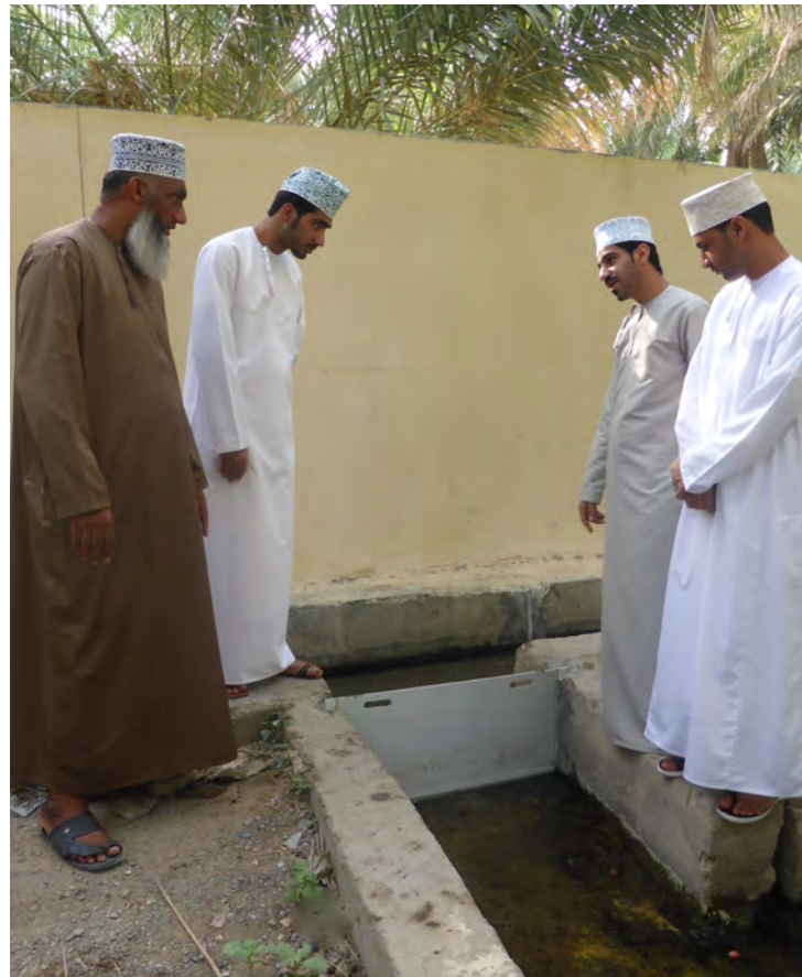
The design of the fibreglass gates was modified several times. The different designs were each tested in the falaj.
