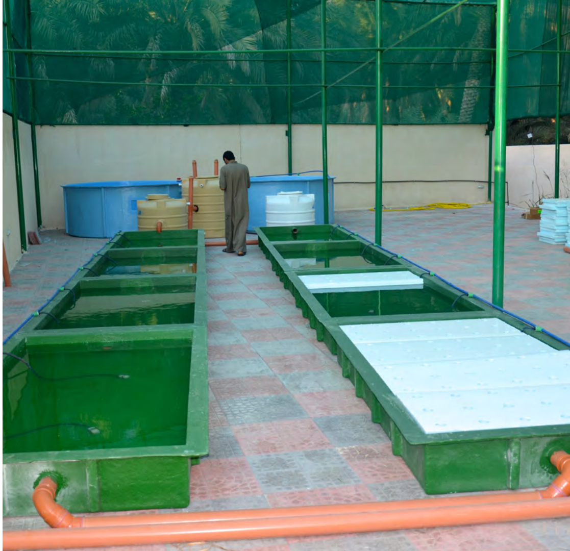
The newly installed water troughs and fish tanks in the shaded enclosure built to house the Luzugh aquaponics unit.
