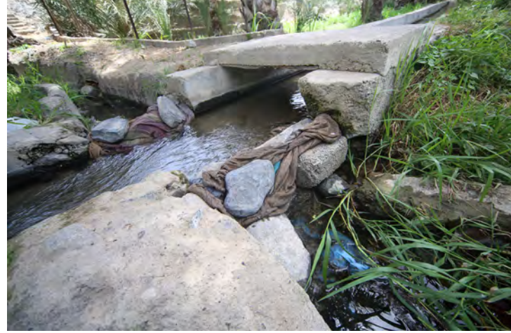
A lot of water was being wasted because of leaking falaj gates, blocked with stones and rags. The wakils were keen to reduce the water loss.
